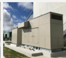
Emergency private power generator
